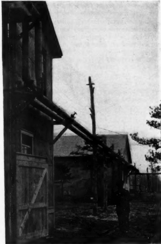
TERMINUS OF BRANCH LINE HEATING MAIN ENTERING BUILDING
