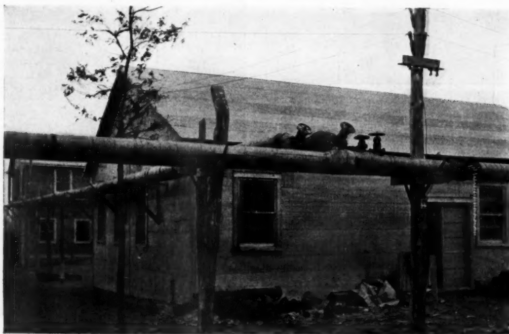
TRUNK LINE HEATING MAIN SHOWING EXPANSION JOINT, BRANCH LINE AND CROSS CONNECTION OLIVER LOADING COMPANY, OLD BRIDGE, NEW JERSEY
