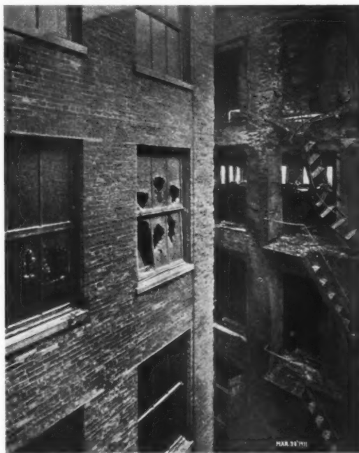
THE ASCHÉ BUILDING FIRE Holes made by firemen by pushing nozzles of hose through wire glass, which served as a shield to fight fire across the court
