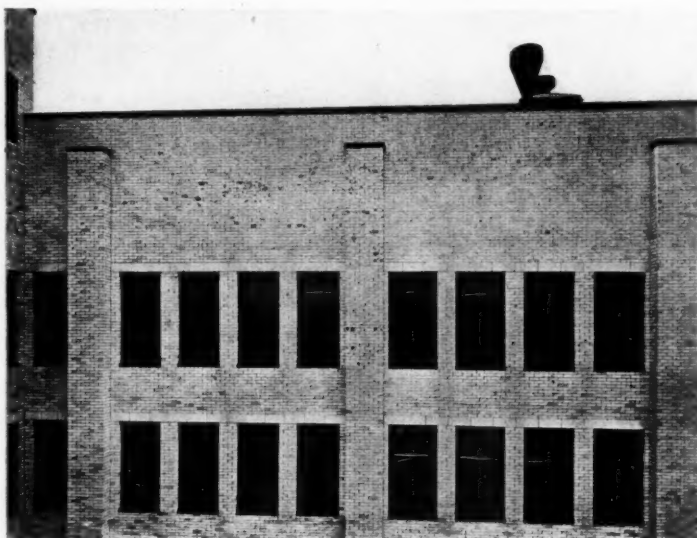
WALLS IN A COURTYARD, SHOWING EFFECT OF "PEELED" ENAMEL BRICK
