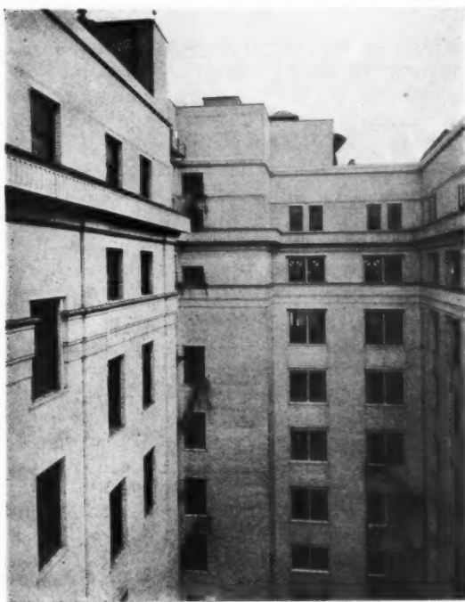
View in court of County Building, Chicago, showing effect of discoloration in enameled brick. The four-inch projection in the wall surface at left, shows a wall surface of enameled brick that will not discolor.
