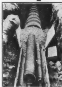
J-M Sectional Conduit after ten years' service.
