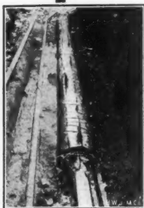
Wood Conduit after one year's service.
