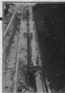
Wood Conduit after One Year's Service
