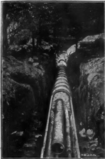
J-M Conduit after 10 years' service
