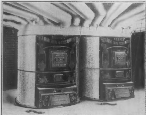
BATTERY OF TWO KELSEY GENERATORS
