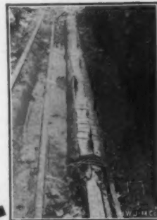
Wood Conduit After One Year's Service
