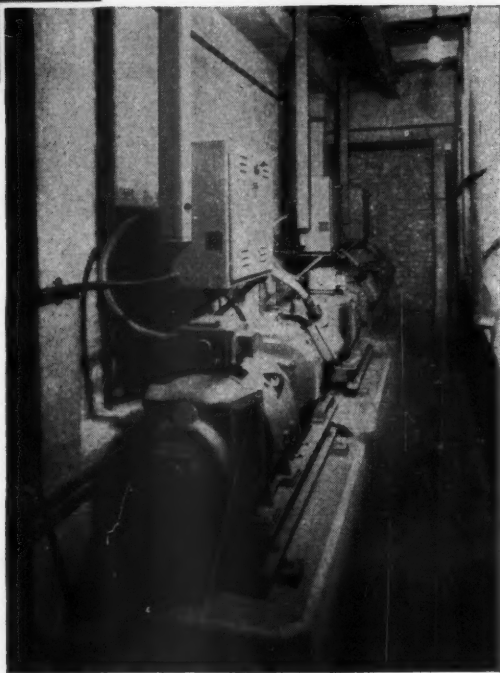
Three of the seven 21 kW motor generator sets associated with each lift installation.
