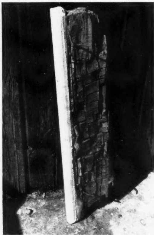
Fig. 2: the bottom of a window board removed during alterations to a house. The window wood is badly affected by dry rot although it did not show on the surface. The house was built about 30 years ago and the back of the frame had not been protected.
