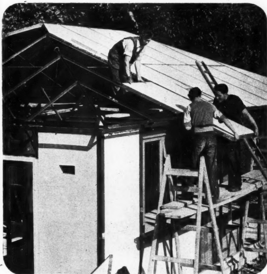
Left, fixing a roof panel in position; the cladding material for both walls and roof is of panelling incorporating a patent compound. Below, sketch of the single storey prototype.
