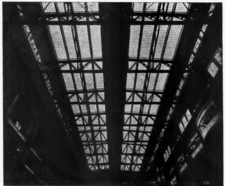
The illustration is of the roof of the turbine house at Fulham Power Station where many thousands of sq. ft. of GLAS-CRETE constructions were installed. The construction shown is double glazed in order to minimise the risk of condensation which is a vital point in connection with electrical machinery.
