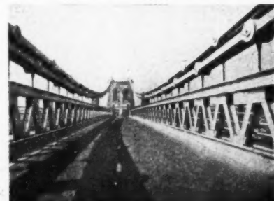
Top, the main span of the old Menai Bridge. Below, the main span of the reconstructed bridge looking towards Anglesey Pier. The character of Telford's design has been retained as far as possible. See No. 2506.
