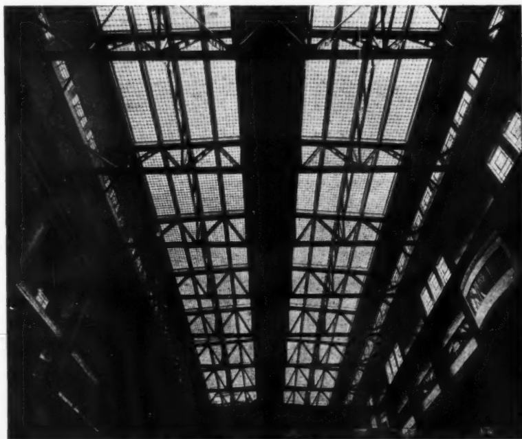
The illustration is of the roof to the turbine house at Fulham Power Station where many thousands of sq. ft. of GLAS-CRETE constructions were installed. The construction shown is double glazed in order to minimise the risk of condensation which is a vital point in connection with electrical machinery.
