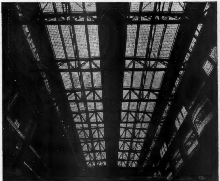
The illustration is of the roof to the turbine house at Fulham Power Station where many thousands of sq. ft. of GLAS-CRETE constructions were installed. The construction shown is double glazed in order to minimise the risk of condensation which is a vital point in connection with electrical machinery.
