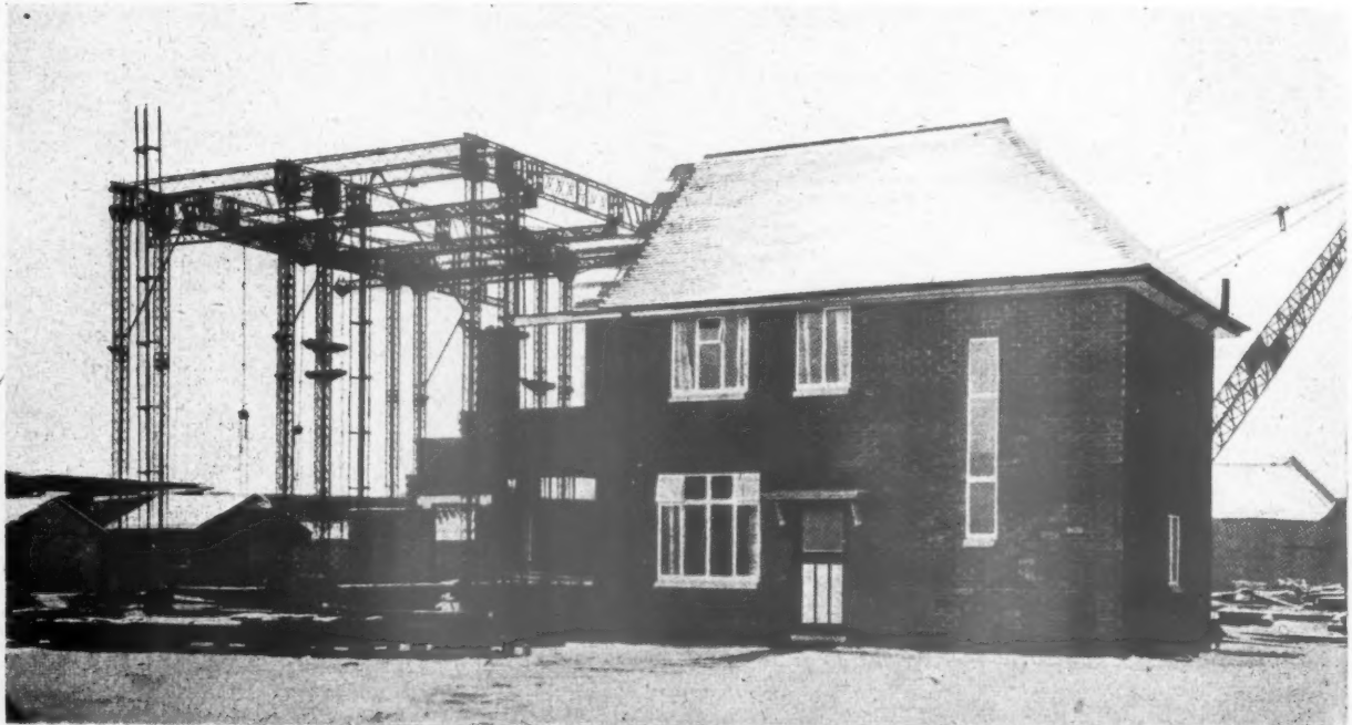
Smith's building system applied to house building. One prototype house is complete; steel gantries are in position for erecting the second house. See No. 1908.
