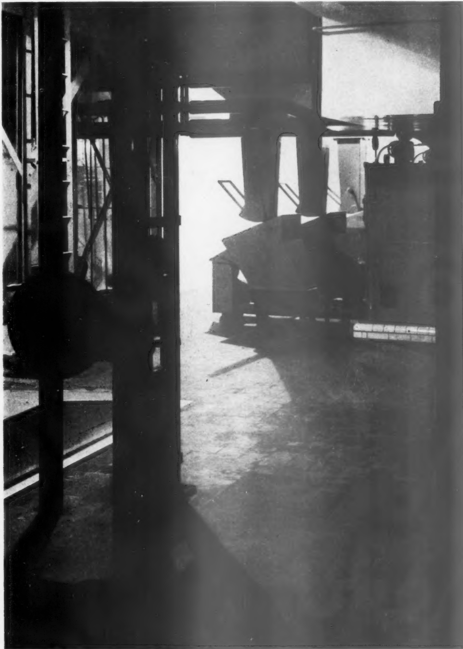
A view in the boiler house
