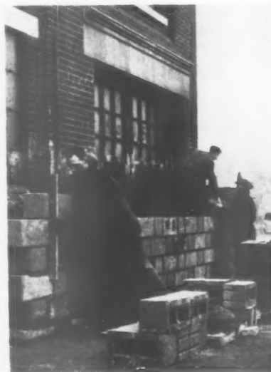
Hollow concrete blocks being erected outside the premises of Hovis in Grosvenor Road, S.W.1.
