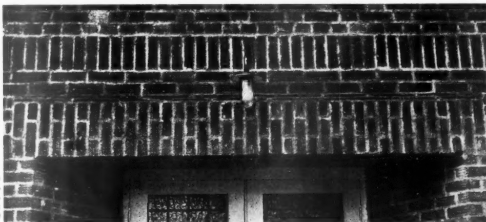
Lintel at Bexley Heath Church and Parish Rooms. Architect: P. M. Andrews, A.R.I.B.A. Contractors: Norman Wright (Builders) Ltd.
