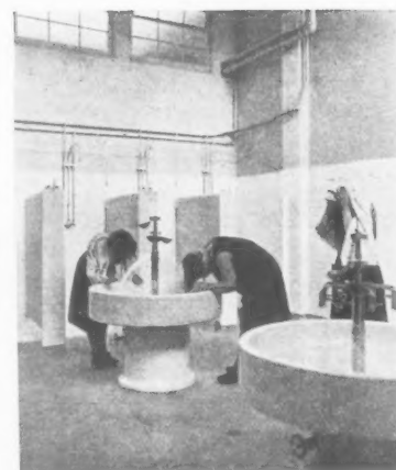
Freestanding washing fountains allow a number of workers to wash at the same time and the water consumption is small.
