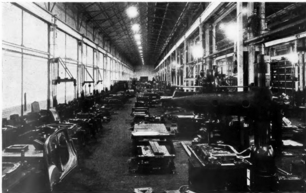
Body panel assembly shop showing small wall cranes on the left and a range of unit heaters on the right.
