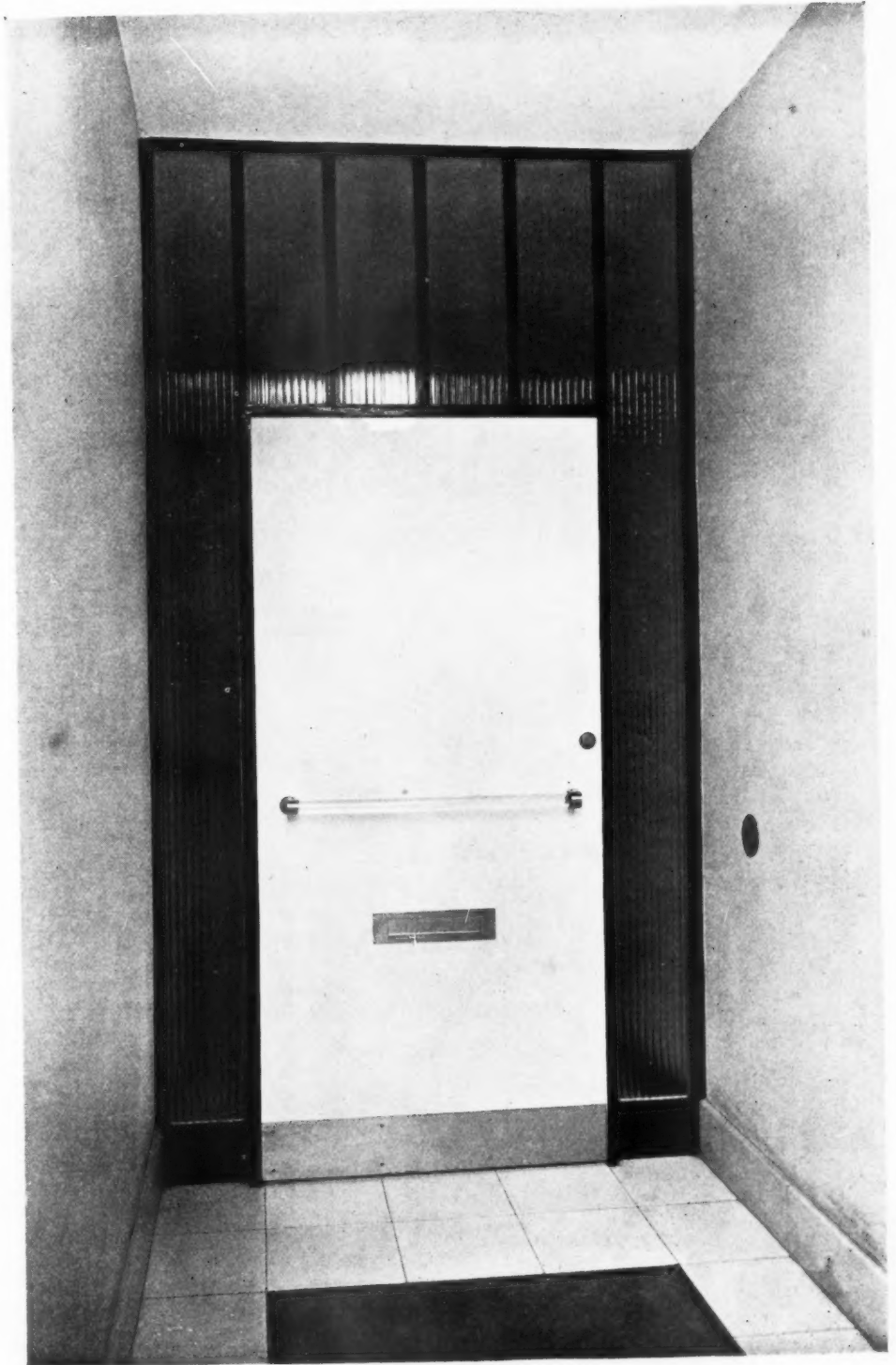
The entrance door is set back in a deep recess ; it is finished with yellow cellulosed metal-faced plywood. The door has a surround of panels of reeded plate glass, and the side walls of the entrance have a rendered finish. Door furniture and kicking plates are in bronze, and the sides of the mat sinking are also finished in bronze. The entrance is paved with buff-coloured tiles. Details are shown overleaf.
