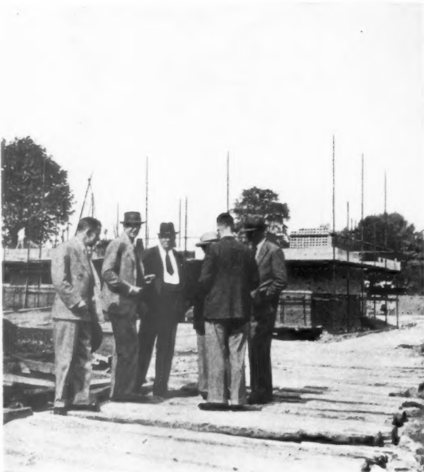
On the job: the architect of the new working-class housing estate now being built at Loughborough Park, discussing progress with his assistants and representatives of the builders. From right to left: Messrs. E. W. Armstrong (architect); J. K. Dale—back view (of C. Miskin & Sons, the contractors); hat—J. Ball (general foreman); C. J. Elms (clerk of works); J. W. Rivett (architect's office) and H. J. Hall (architect's office).
