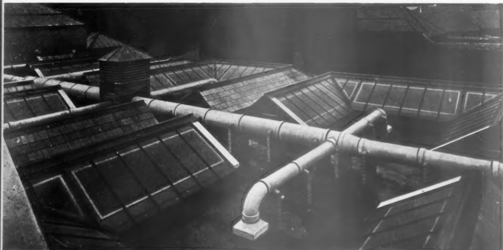
General photograph showing asbestos cement duct work installed on the roof of the existing building.
