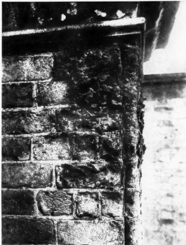
A red-brick pier at Chelsea Hospital, showing the exfoliation.
