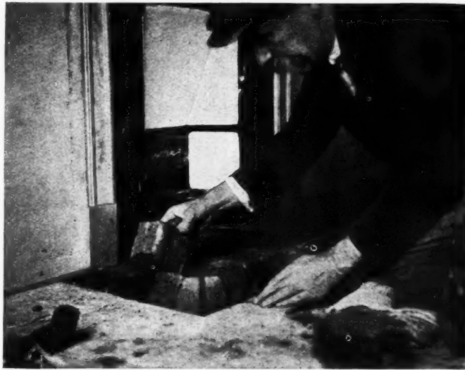
Above (left), figure two. The bricks were marked for cutting by means of a process of application to their positions, and (right)—figure three—cutting the bricks to a tapering shape with an old-fashioned double-ended scutch. Below, figure four. The four tilted bricks at the corner of the curb have to be cut to form the mitre. They are shown placed loosely in position while adjoining bricks are first set.
