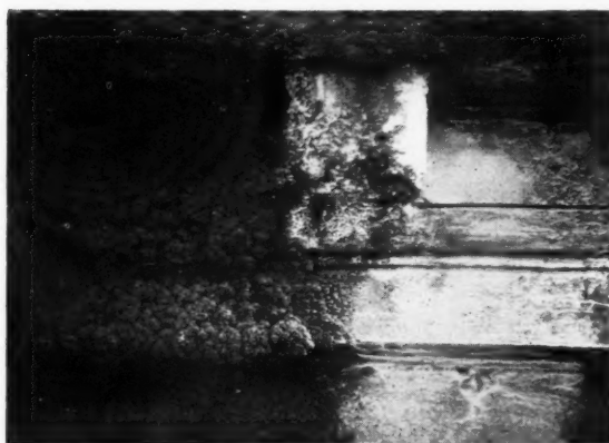
A Portland stone cornice at Somerset House. A near view showing the encrustation, and a portion with the encrustation removed.
