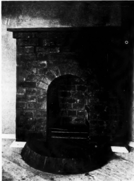
Figure one. Fireplace in a subsidy cottage. Wide radiating joints were designed, but the bricklayer insisted upon cutting the bricks to give parallel-sided joints in the curb.
