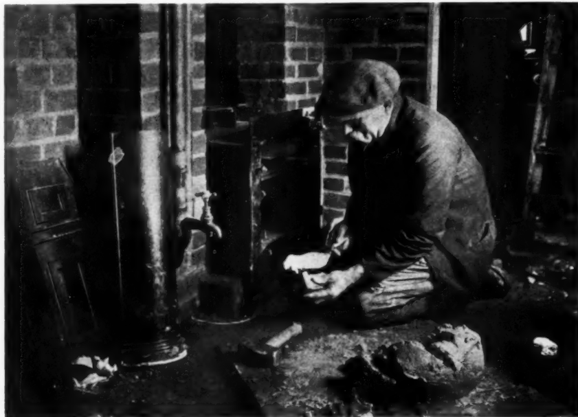
Above, figure five. Forming the side of a flue. The brick is being placed on its lime mortar bed. Below, figure six. Building up the vertical side of the oven flue. The quadrant plate of cast-iron will ultimately cover up this brickwork.
