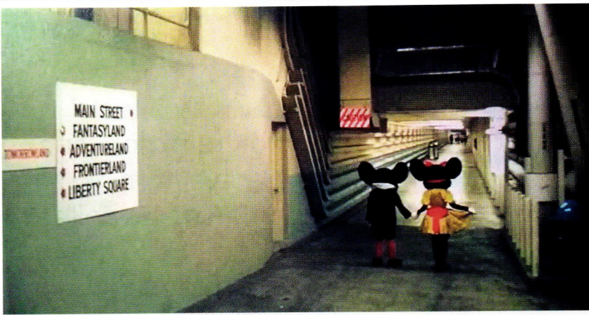
The utilidor at Disney World was built in the late 1960s. It houses utilities, is used to transport goods, and includes walkways for employees to move around the park.
