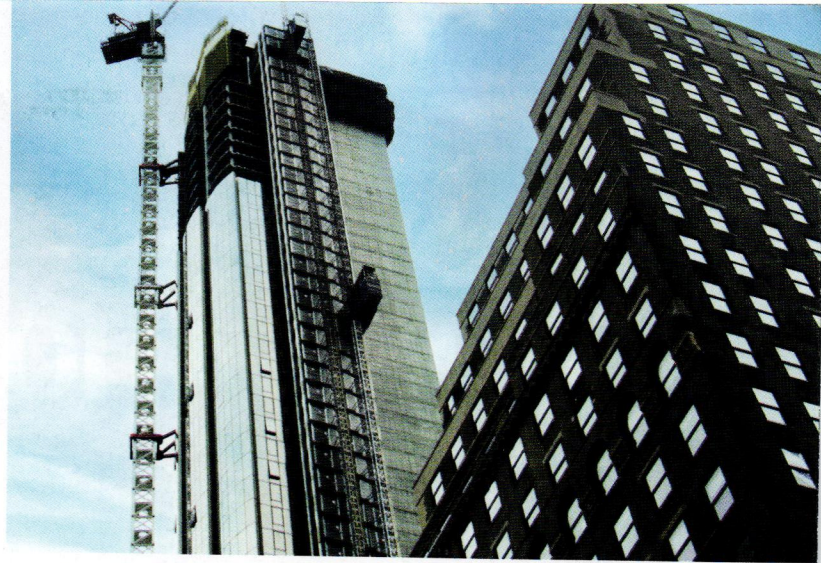
989 6th ave, New York, New York, where Siderise CW-FS Firestop and CW-CB Cavity Barrier are being installed
