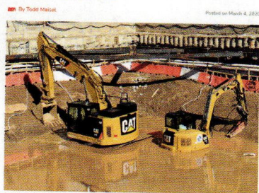
A 24-inch water main broke early this morning on North 6th Street and Driggs Avenue, flooding basements and a construction site, while causing the street near the L train construction to crack and undermine. (Photo by Todd Mattai)
