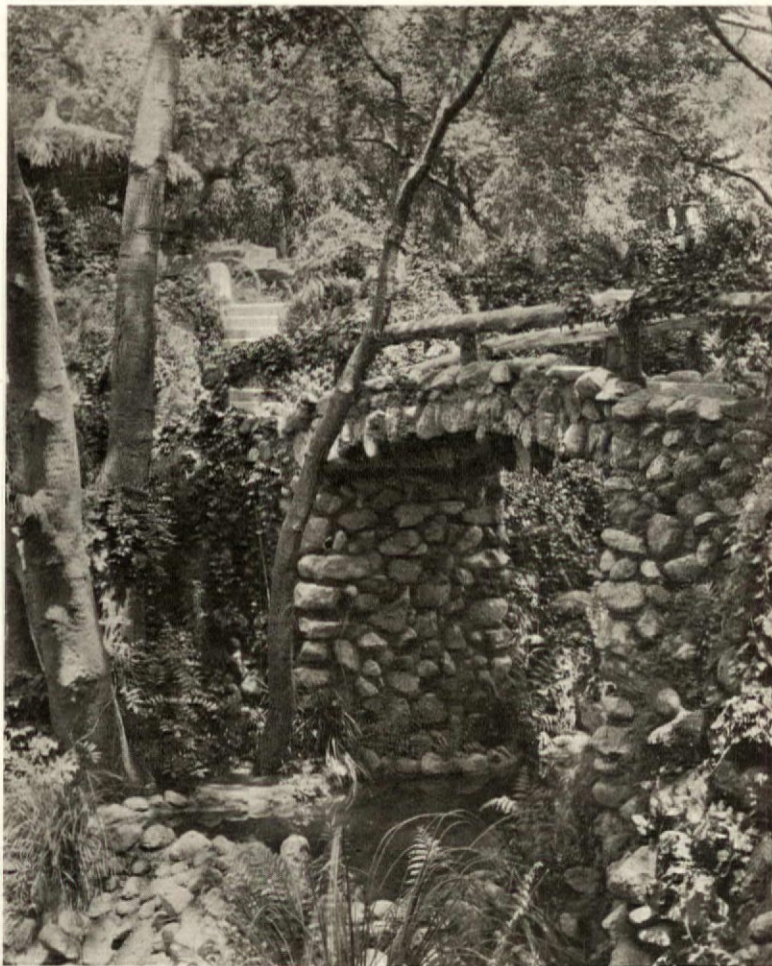
A stone arched bridge with a rail of rustic wood which forms a picturesque safeguard
