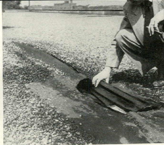
14 lbs. per sq. ft. of upward pressure are needed to separate the plies of a built-up roof, but there is no measure of the shearing effect of blisters between plies. Above, the scars which blisters leave.
