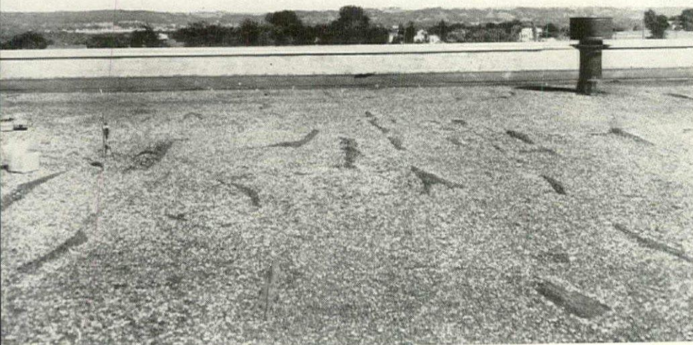
Typical buckling and erosion caused by blisters
