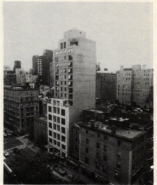
Thierry W. Despont and Emil Steo. 1080 Madison Avenue under construction. (photo: Gaston Dubois)
