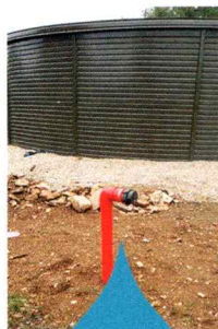
FIRE DEPARTMENT CONNECTIONS
