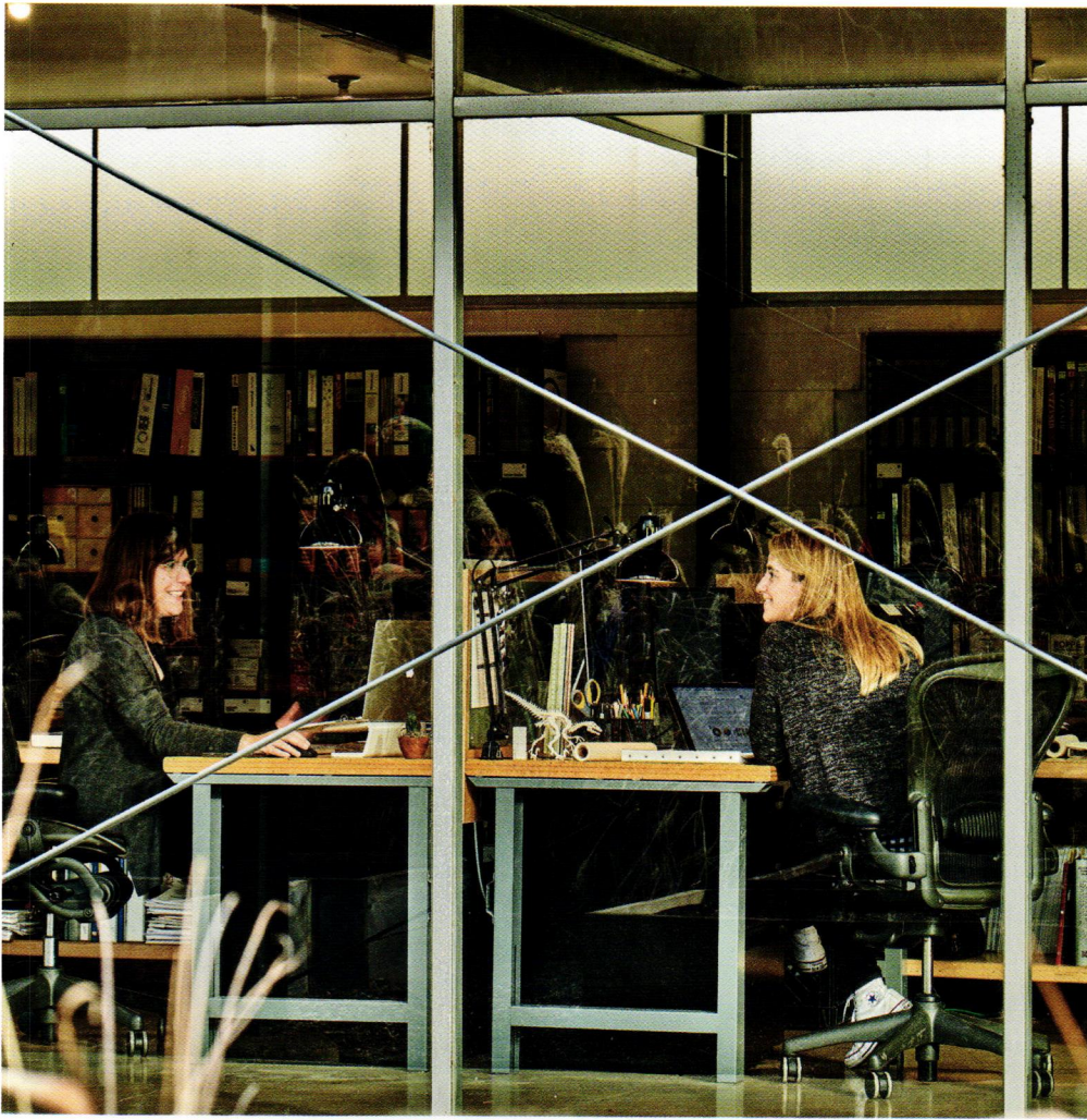
A CMU screen wall was removed, opening the glazed interior to the garden.
