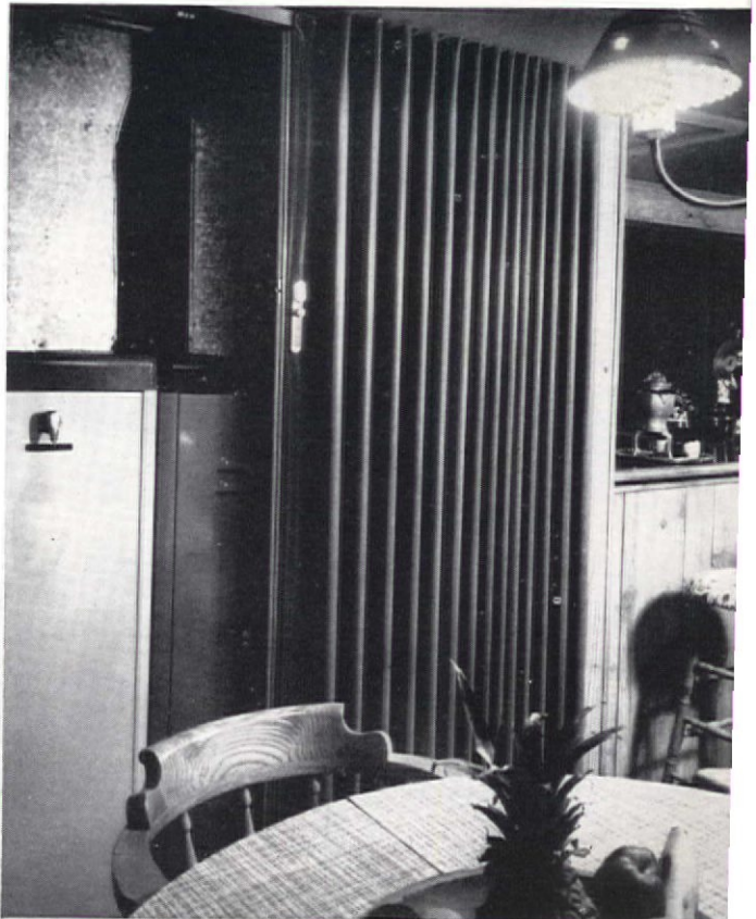
This ingenious folding panel conceals the heating plant, fitted neatly into space behind the bar. Guests never know it's there until it's pointed out to them
