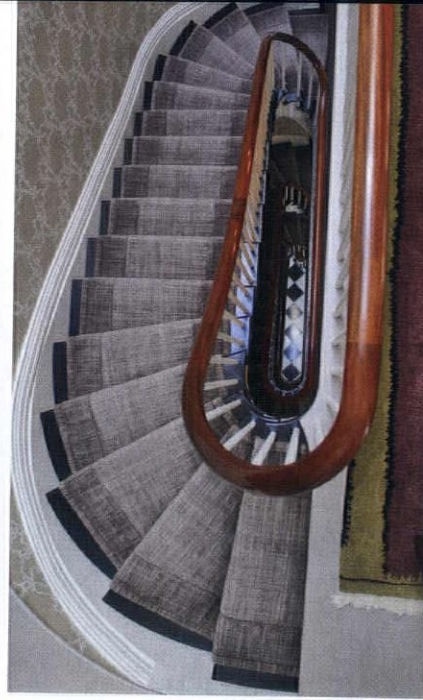
FAR LEFT Although the treads and risers don't meet modern building codes, early staircases like this Federal-era example are so compactly built, they tend not to settle as much as later stairs. LEFT Narrow and compact, cylinder stairs in a restored staircase on Boston's Beacon Hill are common in row houses built before 1840. BELOW Dogleg stairs use landings wherever the stair turns, making them compact and easy to climb.
