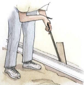
A longer pry bar offers more leverage. Protect plaster, as here with a shim (shingle).
