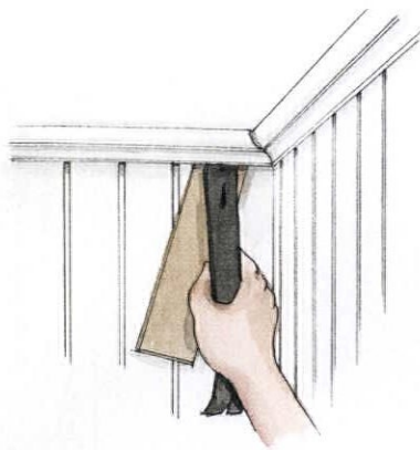
The coped piece—installed in the corner after its mate—must be removed first.
