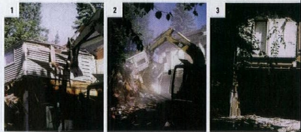
BEFORE Part of the previous kitchen and a breakfast area were inside the bland 1970s addition. ABOVE Demolishing the boxy addition exposed the original rear wall.
