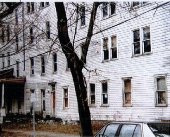
▲ Clapboards and windows that sag like a clothesline may indicate foundation or sill problems.
