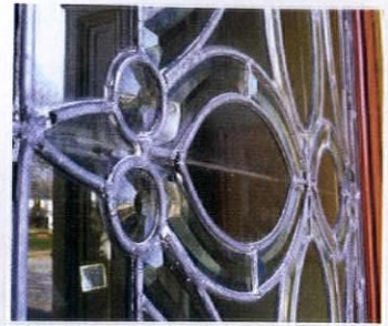
FAR LEFT: The upper window needs glass replacement. LEFT TOP: A transom damaged by high winds is in need of glass replacement. LEFT BOTTOM: This panel suffers from brittle waterproofing putty as well as buckling. MIDDLE: Notice the broken solder joints and bulging in this zinc-channel door panel; it will need to be removed to repair it. ABOVE: This leaded door panel suffers from broken solder joints and loose waterproofing putty.
