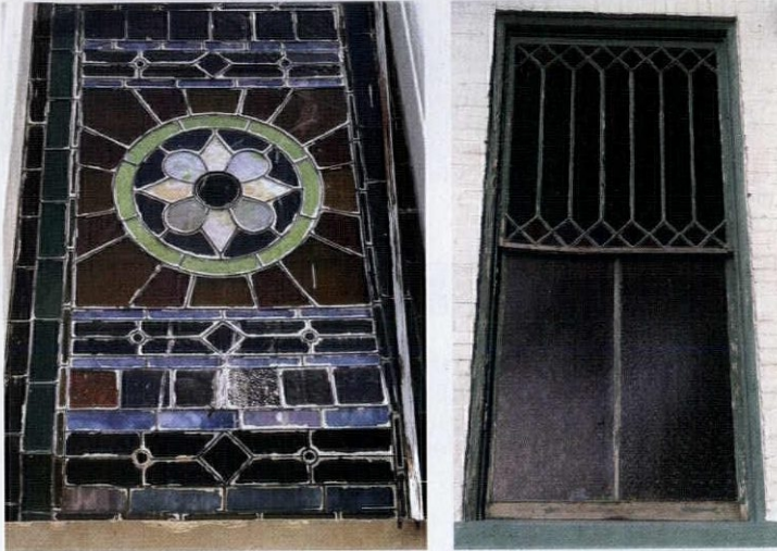
LEFT: Deferred maintenance and inadequate past installation results in this condition. RIGHT: Evidence of deteriorated wood and window sash.
