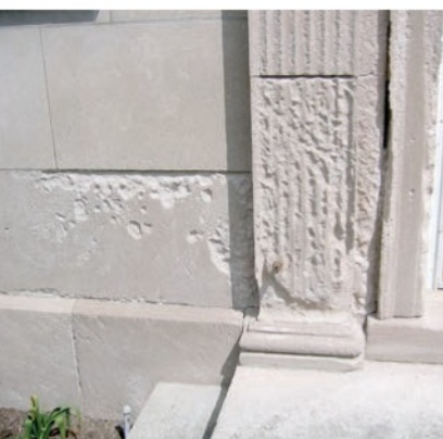
"I have pictures of the birds caught in the act," writes the homeowner, describing pecking damage in the limestone around two entry doors.
