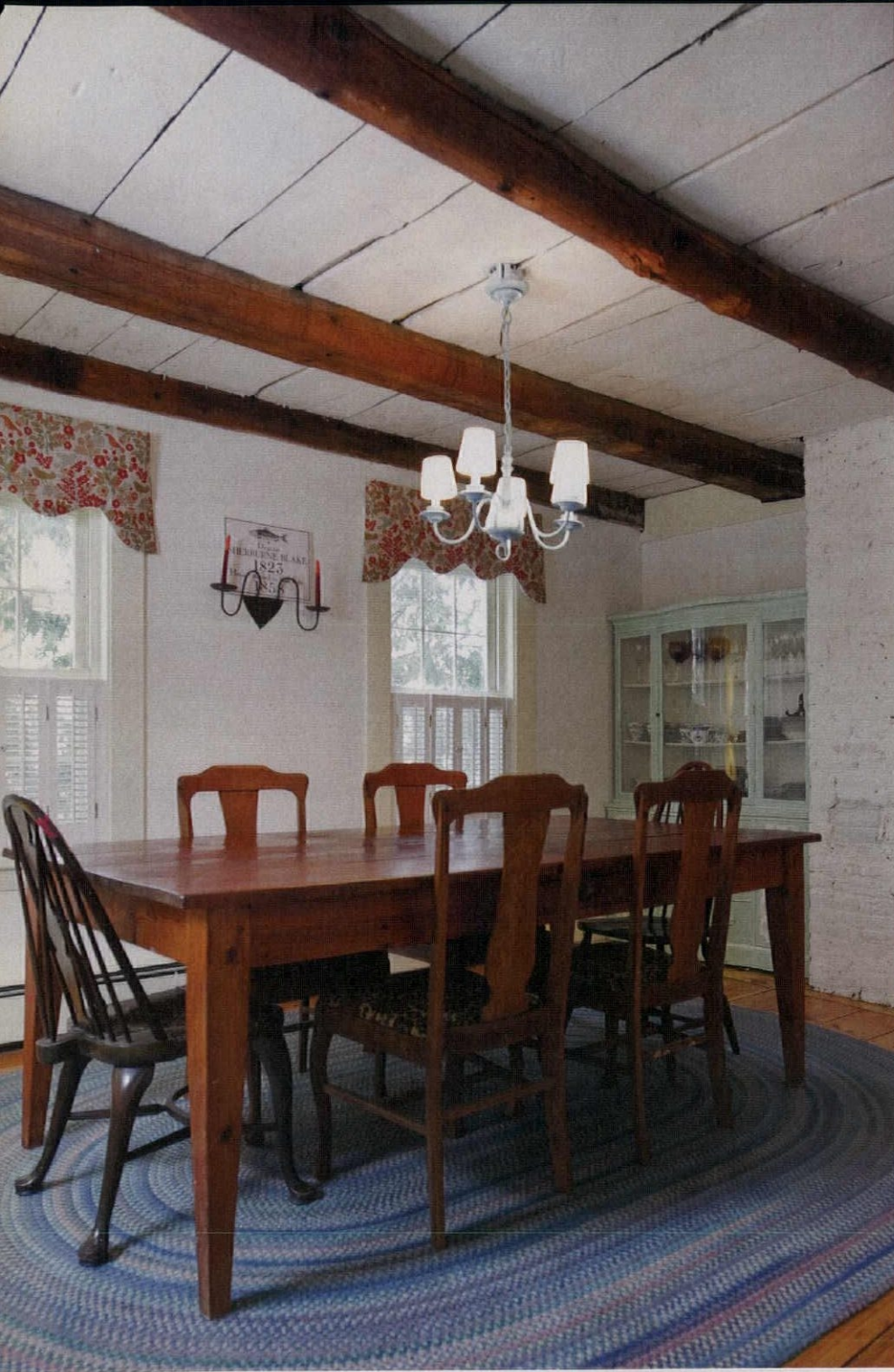
LEFT: Exposed beams in the dining room offer clues to the house's original configuration. ABOVE: Scabs are visible on some beams, which were cut to modernize the house.
