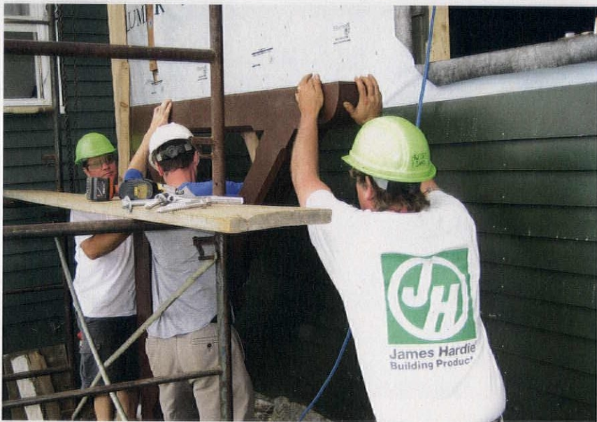
ABOVE: Workers prepare the structural members of the house (top) to receive new and restored piazza brackets (bottom).
