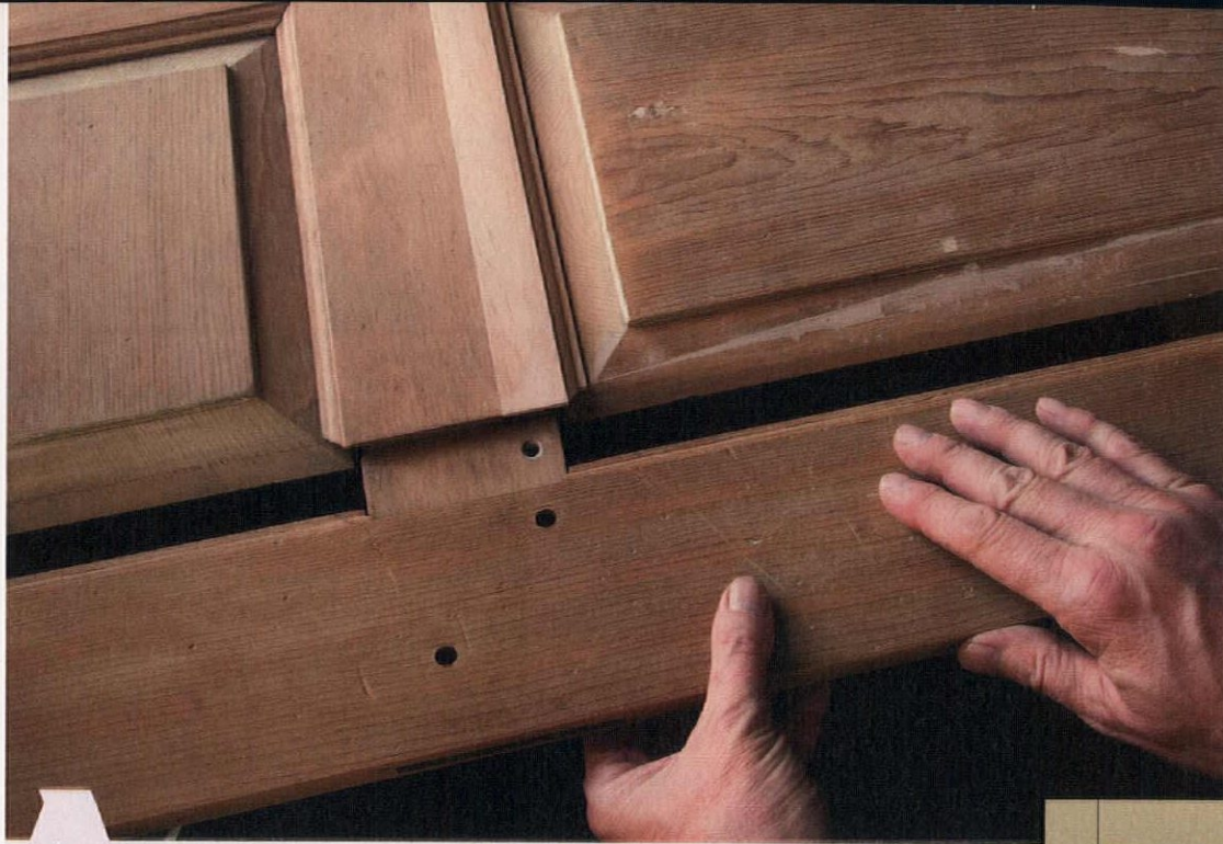
OPPOSITE: Six-panel doors are common on Federal, Georgian, and Colonial Revival houses, such as this 1938 Colonial Revival on Cape Cod. LEFT: Repairs often require disassembling and reassembling the door.
