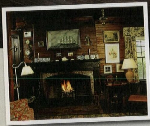
ABOVE: Thanks to the leaking chimney, the original pine mantel was suffering from rot.
