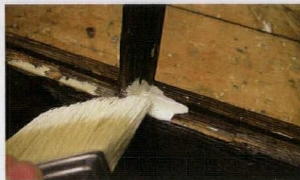
Puddling the primer at each joint helps it soak in and seal the end-grain.
