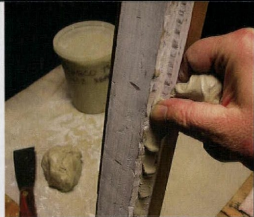
A solid "bed" of putty in the sash's glazing rabbets helps seat the pane of glass.
