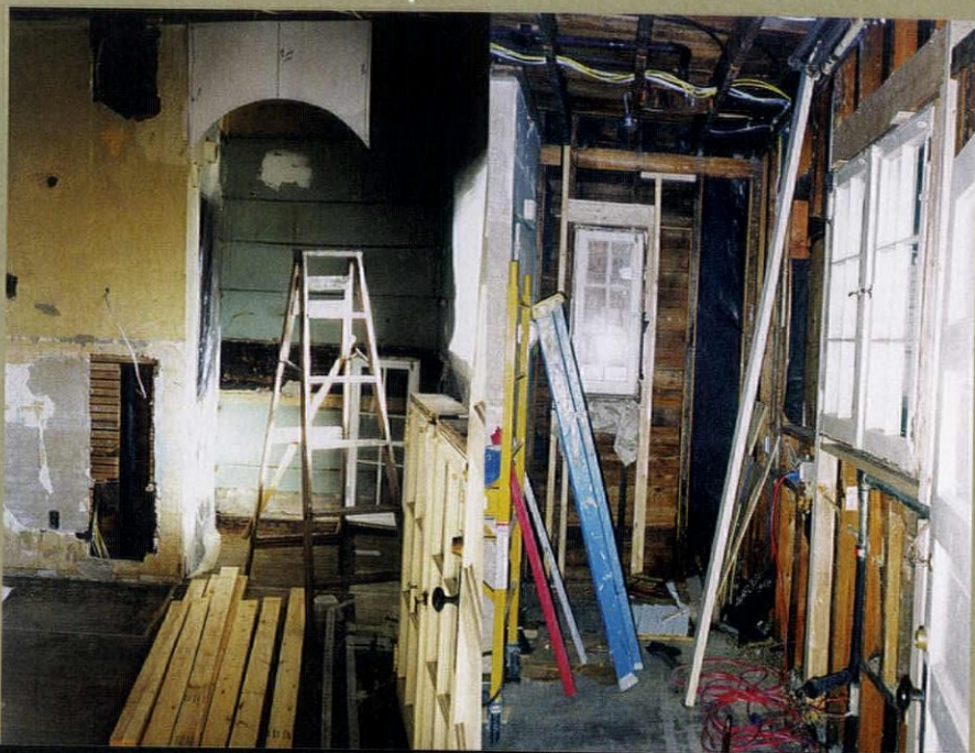
LEFT: Upon dismantling the kitchen, Ryan and Montana found ghosts of original butler's pantry shelving (visible on the back wall below a mock-up of the new passageway). RIGHT: The layout of the pantry was reconfigured to add a salvaged casement window to bring in additional light.
