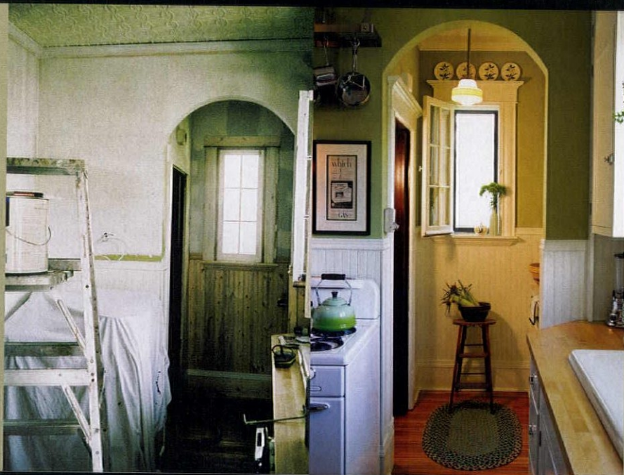
LEFT: The dimensions for the new passageway between the kitchen and pantry were based on a ghost Ryan and Montana found under the carpet. RIGHT: With beadboard wainscoting and a reproduction light fixture, the new butler's pantry pays homage to the original space.
