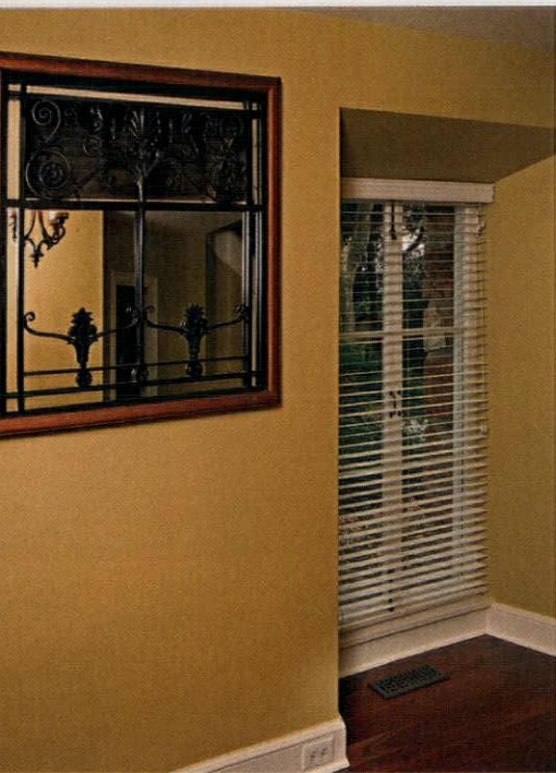
ABOVE: Air-return grilles are incorporated into the home's décor. TOP: The kitchen and dining room were in such poor shape that they had to be completely redone, allowing the Neiblumns to run ductwork under the floors.
