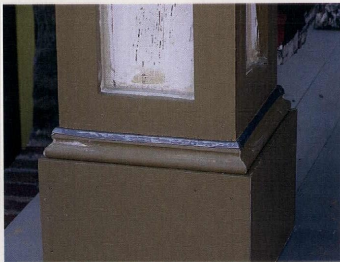
ABOVE: When joints at the base of square columns point downward and are protected by flashing, rainwater naturally slides off the wooden element, preventing infiltration that can lead to rot.
