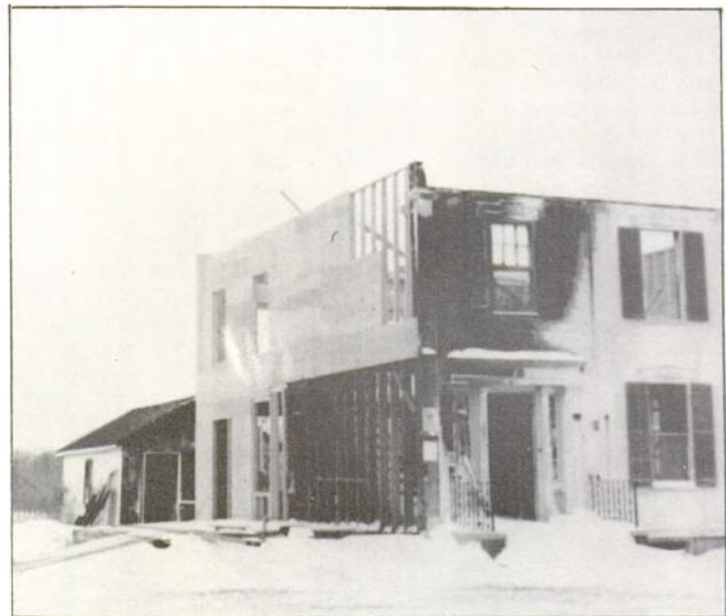
The house now shows the rebuilt portion, with the pediment removed for copying and salvage. The heavy bracing and stud-work is original.
