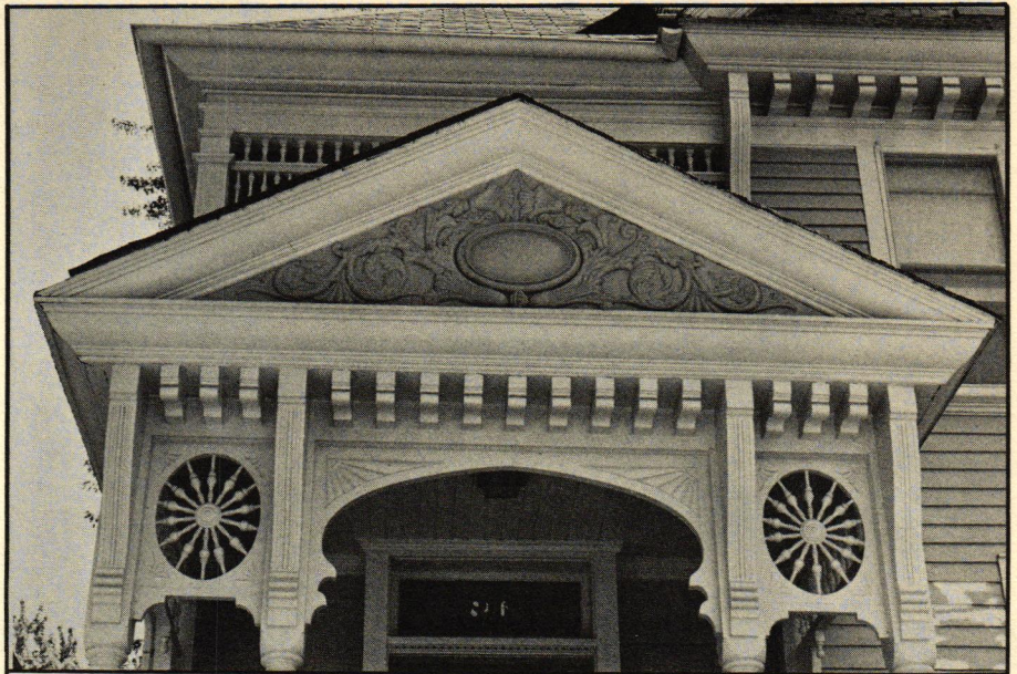
A striking feature of the porch is the embossed panel set into the pediment. Although it looks like carved wood, it is actually stamped metal—undoubtedly ordered from an architectural parts catalog of the 1880's.
