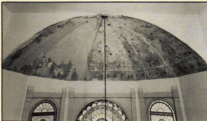
Stencil design on ceiling of bay is being restored. Original cast iron stair light hangs from large gilt star in center.
