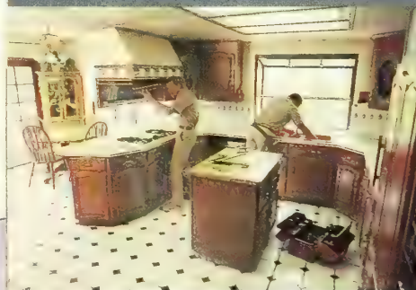
Professional kitchen planning, design and installation.
