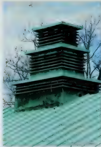
Triple-tiered copper chimney cap, louvered for updraft.
