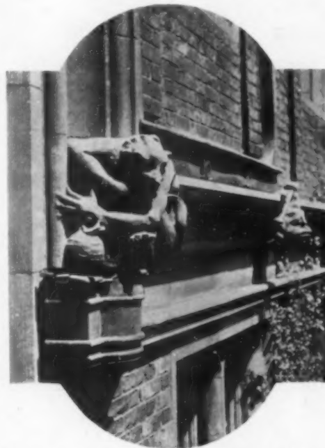
The rain-water head can be successfully used in conjunction with a gargoyle or grotesque
