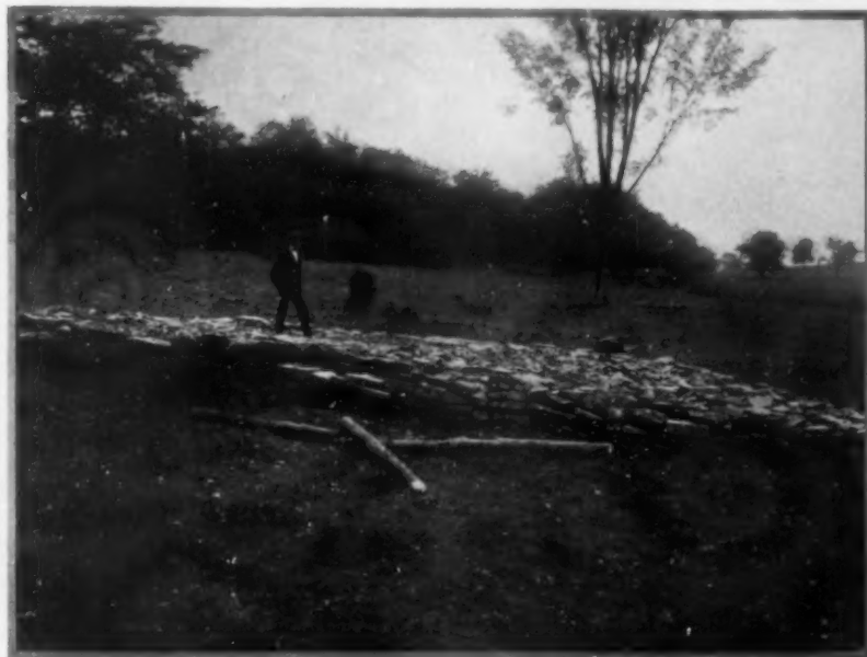
At this juncture the road bed was ready for the dirt, which was laid on a foot thick—a costly item in the bill
