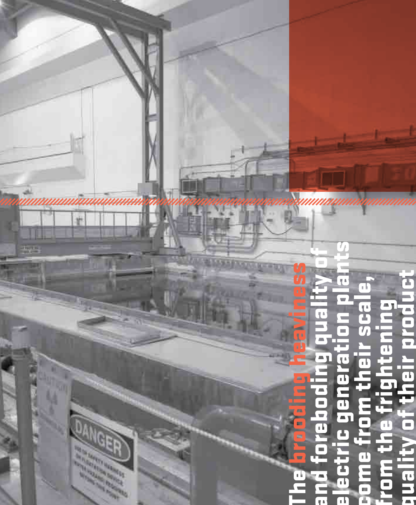
LEFT: Spent fuel storage pool.
