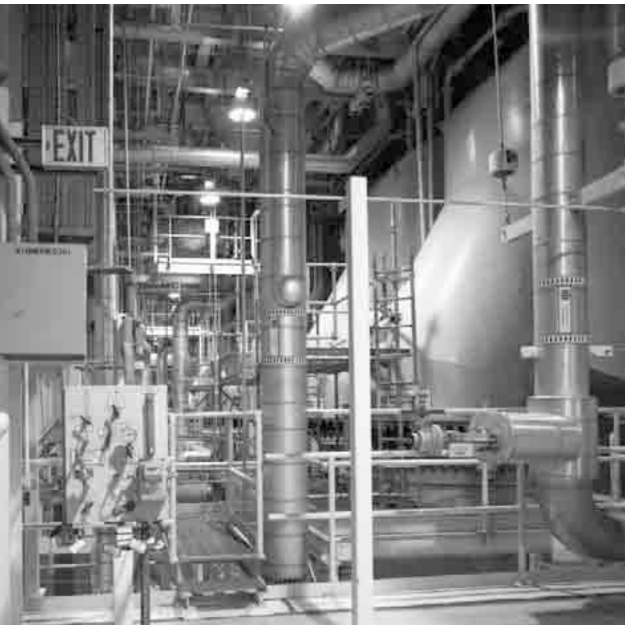
TOP: Machinery and guardhouse on the roof of Unit 1, Turbine Building. ABOVE: Inside the Turbine Building.
