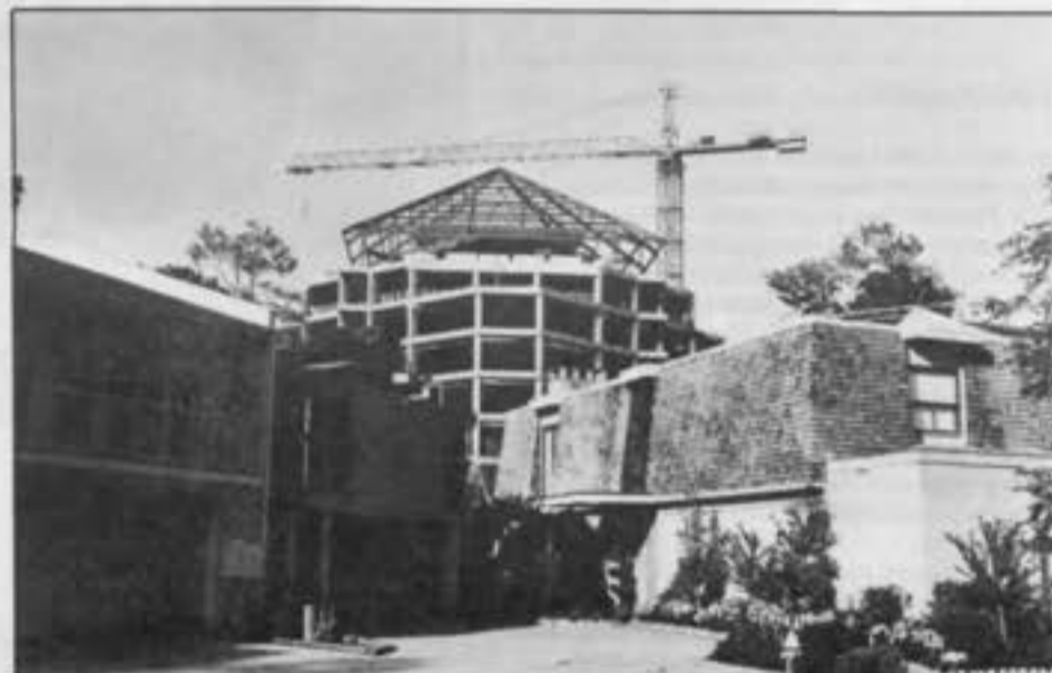
The Park Laureate, under construction, 1985. Howe/Reb Associates, architects (Photo by Paul Hester)
