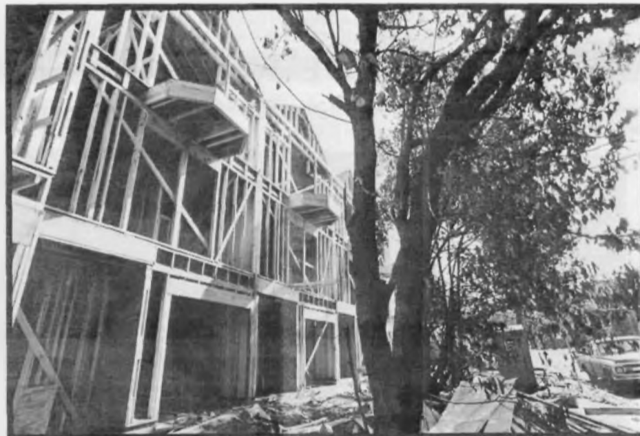
Portsmouth Townhomes, under construction, Alan E. Hirschfeld, architect. A project built after the development ordinance went into effect. (Photo by Paul Hester)
