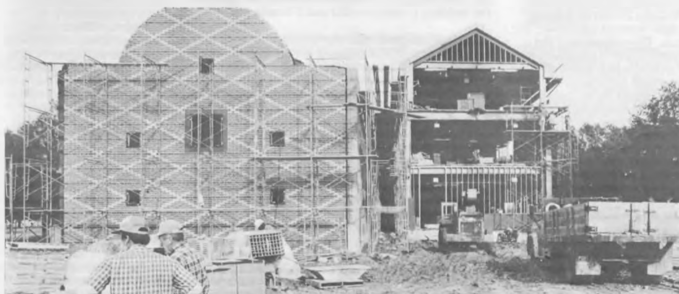
Herring Hall under construction, Cesar Pelli and Associates, architects (Photo by Paul Hester)
