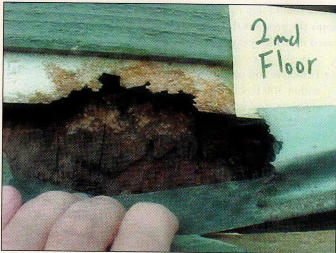
Premature decline. On a beachfront home in Virginia, no Z-type flashing was installed over the ledger-to-house connection, which led to extensive decay.
