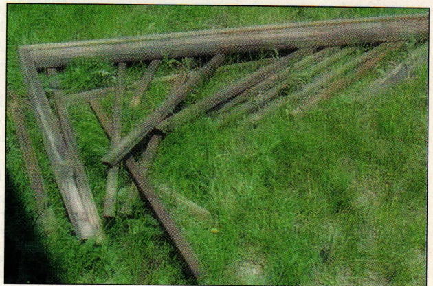
Deadly rail. The photo above shows an example of a grossly deficient guardrail system that produced a fatality and another injured party. In this case, a young man died after falling through the guardrail with posts that were nailed only to joists on the end of the deck. Note the notched 4x4 posts — a detail that is not permitted in the DCA6.
