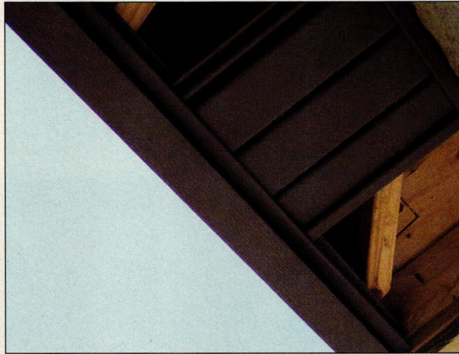
FIGURE 5. The perforations in Alcoa Hidden Vent are recessed in the panel grooves. The manufacturer claims this design provides plenty of ventilation airflow, but when combined with a fascia that extends a full inch below the soffit, the potential for water sheeting off the roof and getting driven by wind or surface tension into the vent openings is greatly reduced as well.
