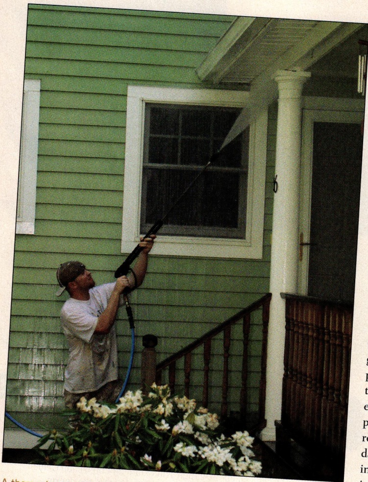
A thorough and vigorous washing is the best prep for routine repainting. Don't neglect the areas under eaves — they can accumulate salt and grime deposited by moisture rising up from soil around the building.
