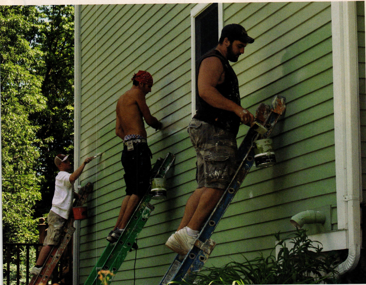
Three painters work together on the shady side of a house to get the paint on quickly. Modern acrylic paints and stains tend to dry quickly compared with older, higher-VOC formulas.
