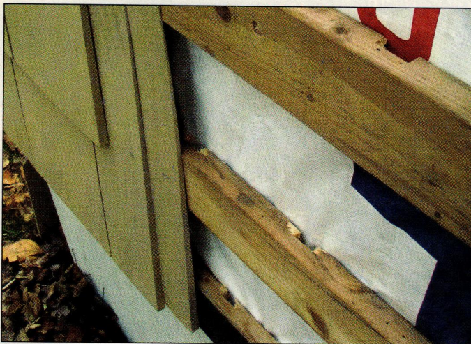
FIGURE 1. The author's first experiences with venting shingles relied on back-kerfed 1x3 furring strips. These back kerfs are essential for allowing water to drain out and air to flow between the horizontal strips, but cutting the kerfs with a dado blade in a radial arm saw proved too labor intensive.
