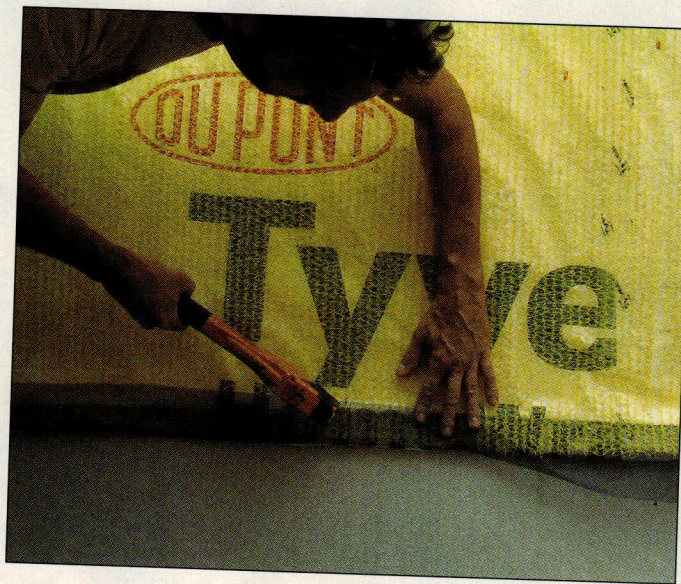
FIGURE 3. Wasps and hornets love to build their nests in the vent space of any rain screen, so exposed edges (at the bottom and top of walls and over windows and doors) must be protected with screening.
